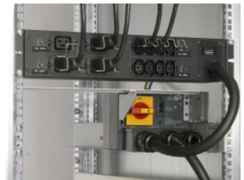
Structured cabling, reliable connection.
