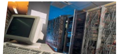
Perfect for high density server enclosures.
